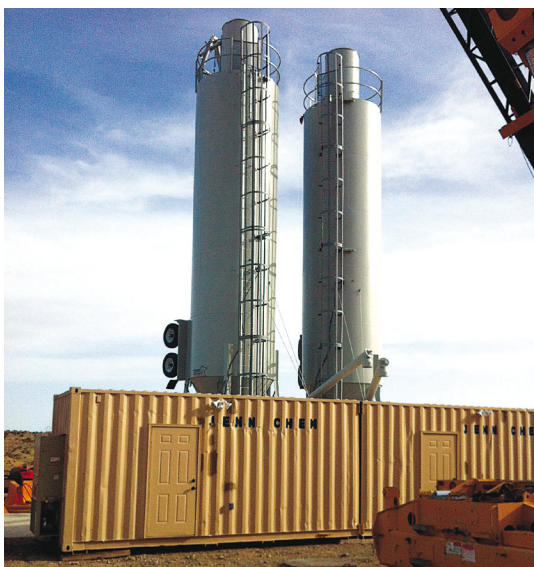
Cement storage silos.
